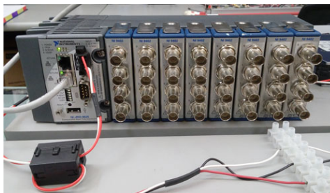
Figure 12 Assembled cRIO with 32-channel digital input.
